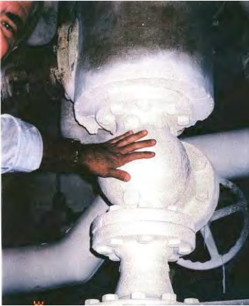
Hot Valve coated with 5 mm for personnel safety
