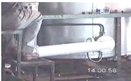
Boiler connector &amp; bend
